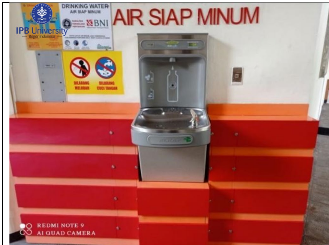
Fig 1. A water station installed next to canteen
