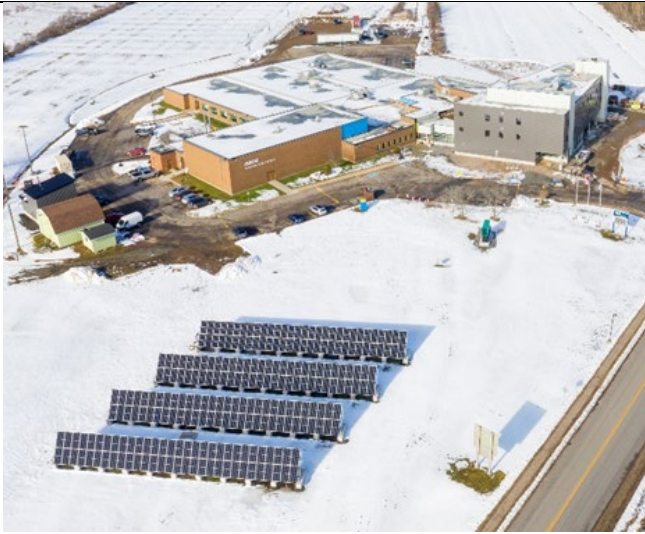
75-Kilowatt Photovoltaic Array at NSCC's Centre of Geographic Sciences in Lawrencetown, NS
