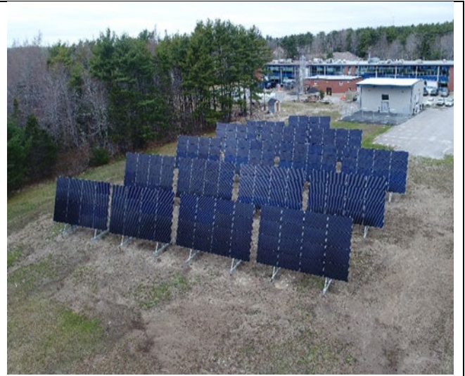
75-Kilowatt Array at NSCC's Shelburne Campus in Shelburne, NS
