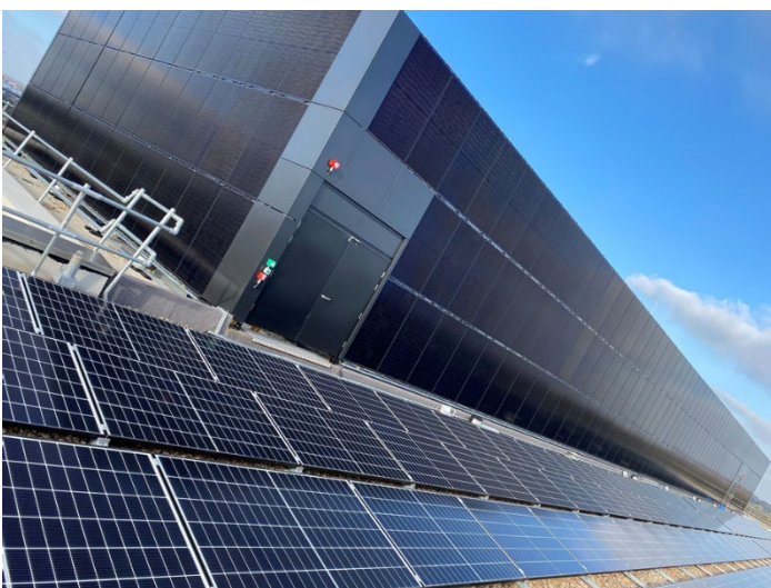
Renewable energy generation and vertical integrated PV on the Interdisciplinary Biomedical Research Building at The University of Warwick
