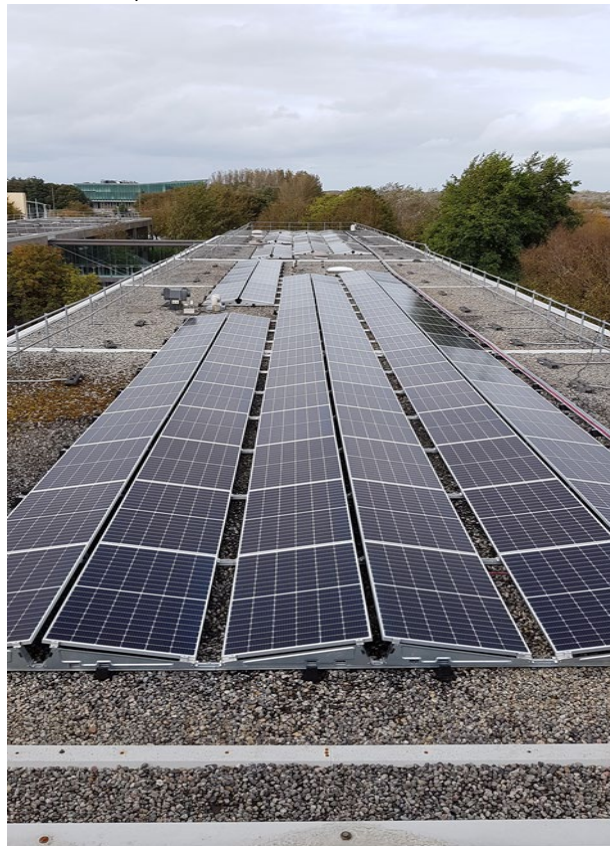
View of PV Installation on Arts Sceince Building at NUI Galway
