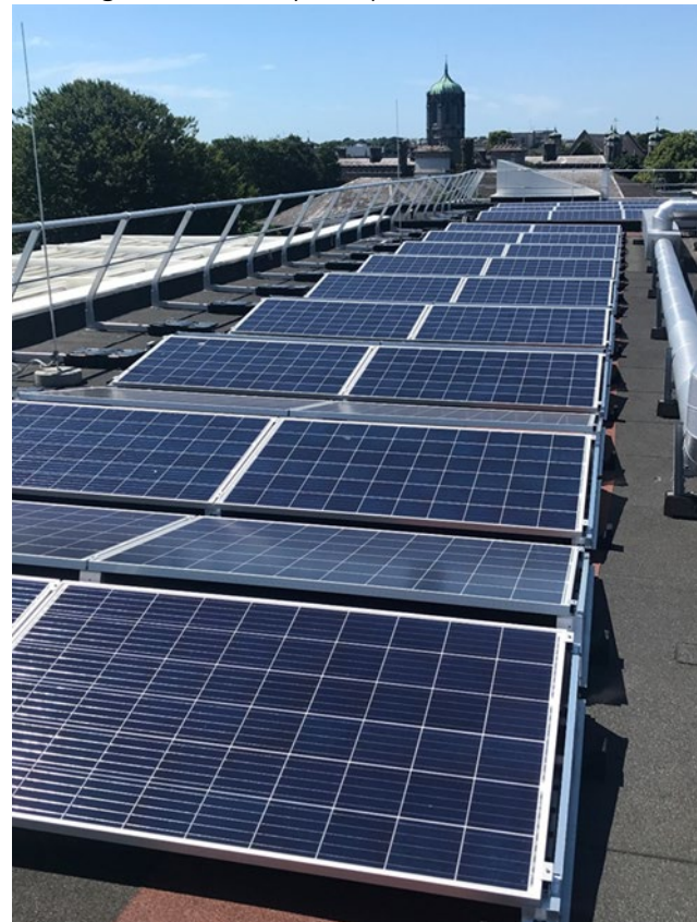
View of PV installation installed on Human Biology Building at NUI Galway Campus
