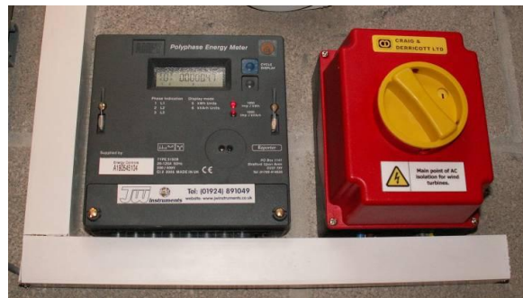
Figure 6 Lockable Isolator and kWh Meter
