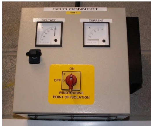
Figure 2 Wind Turbine Controller
