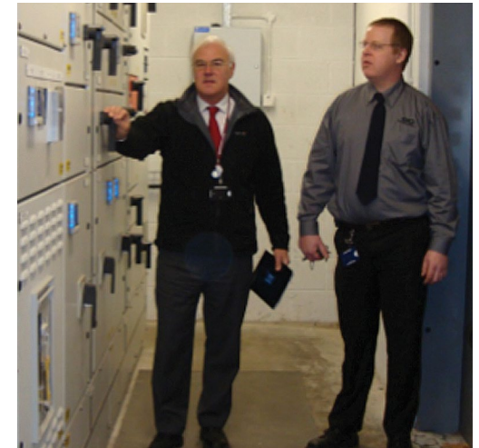
Julian Baxter (left), Estates Director Gloucestershire College with the Head Caretaker, monitoring meters at the main incoming transformer, Gloucester Campus.
