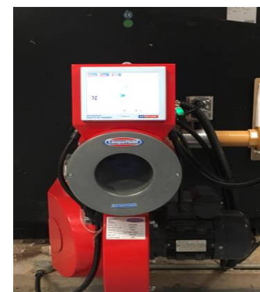
After - new burner
