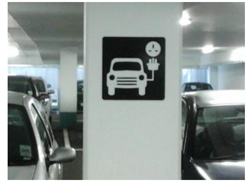
Electric car charging point - BGLZ
