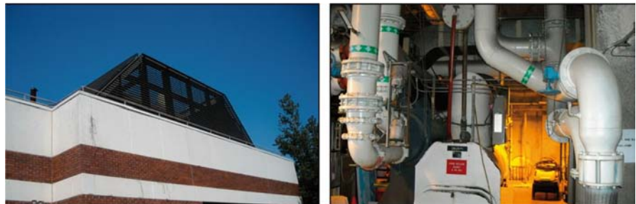
Figure 4. Sutter Medical Central Plant
