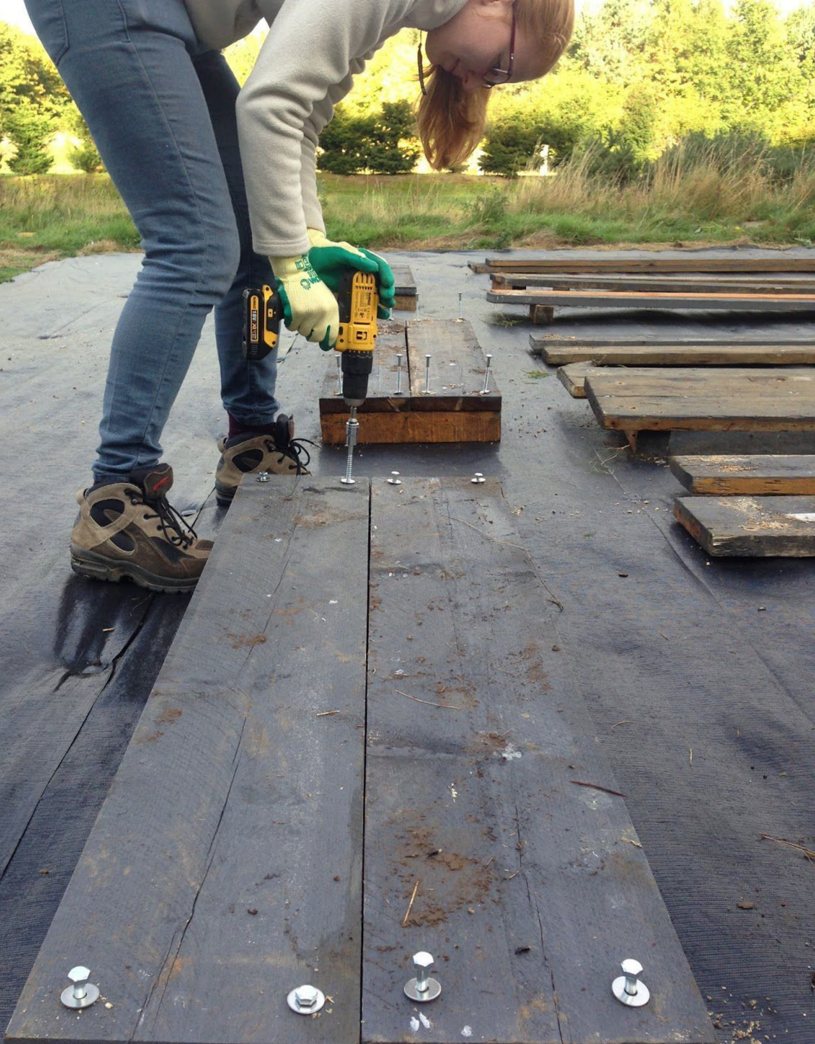
Building raised beds at the Heriot-Watt community garden, where staff and students grow their own fruits and vegetables on campus. Photo: Transition Heriot Watt.
