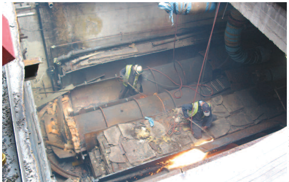
Old Lancashire steam boilers being cut out at George Square Energy Centre in preparation for new equipment installation.
